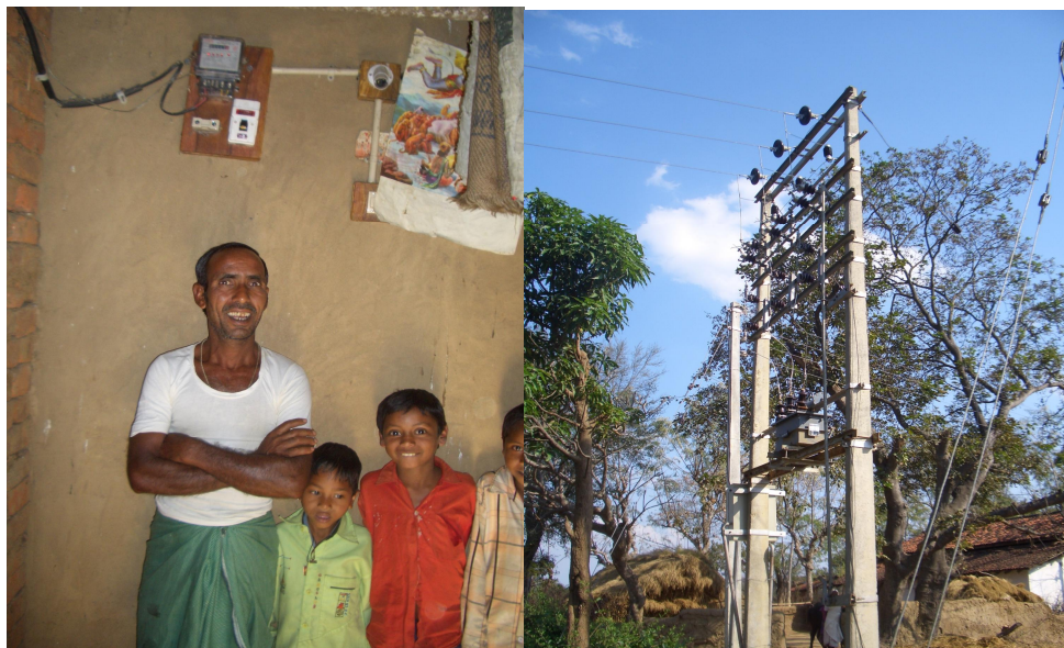
Meter installed in BPL House-hold
